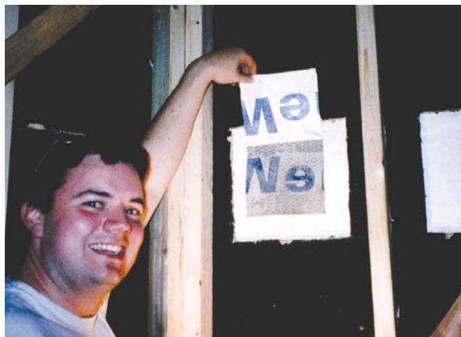
Photograph 6: Hardcoat Stucco Bonding to Plastic Building Paper —A young, happy engineer, discovers that stucco does indeed bond to plastic building papers preventing drainage. The engineer is my friend Chris Schumacher—may he remain this happy when he gets older.
