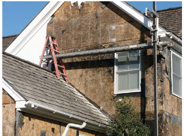
Photograph 4: Hardcoat Stucco Failures —Note that the damage is in the field of the wall away from windows.
