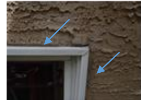
No Head Flashing & Soft Joint
