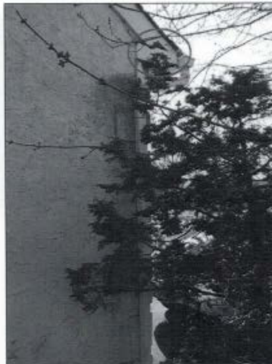
3.0 Item 4(Picture) Moisture damaged wood noted on garage roof returns, replace all moisture damaged wood to reduce the risk of moisture penetration
