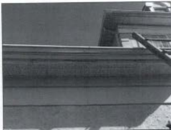
3.0 Item 5(Picture) Replace any moisture damaged wood on fascia
