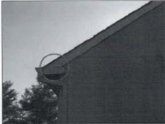
3.0 Item 2(Picture) Moisture damaged wood noted at roof returns on garage, repair as needed to reduce the risk of moisture penetration
