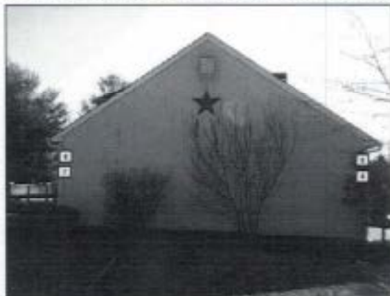
2.3 Item 1(Picture) Left elevation Findings
