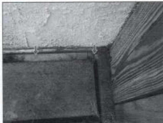
3.0 Item 3(Picture) Rear deck flashing
