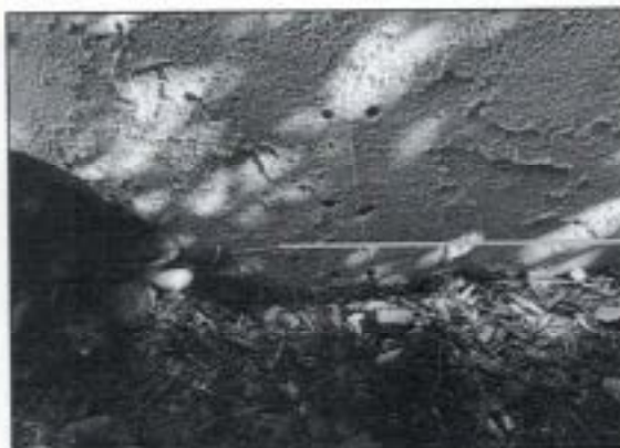
3.0 Item 8(Picture) Foundation wall is slightly above grade, no weep screed is installed, lowering grade to a minimum of 4" below top of foundation wall is recommended to reduce the wicking effects of water & insect activity
